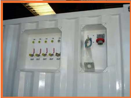
VERSCHIEDENE STROMAGGREGATE ANSCHLÜSSE
