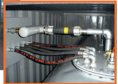
VERSCHIEDENE STROMAGGREGATE ANSCHLÜSSE
